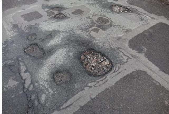
Fig. 7. Photographs of damage (spalling) on section 2.3. Own study
